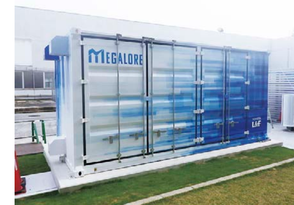
図8 蓄電池 (高浜工場) Fig.8 Storage Battery (MEGALORE ® ) (Takahama Plant)
